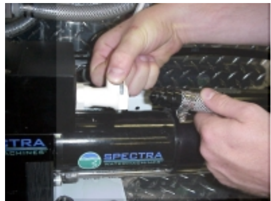
Brine discharge quick disconnect for access.
